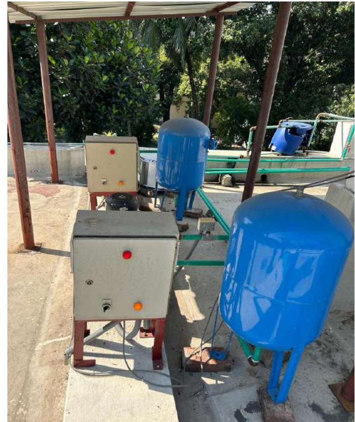
Domestic Booster System
