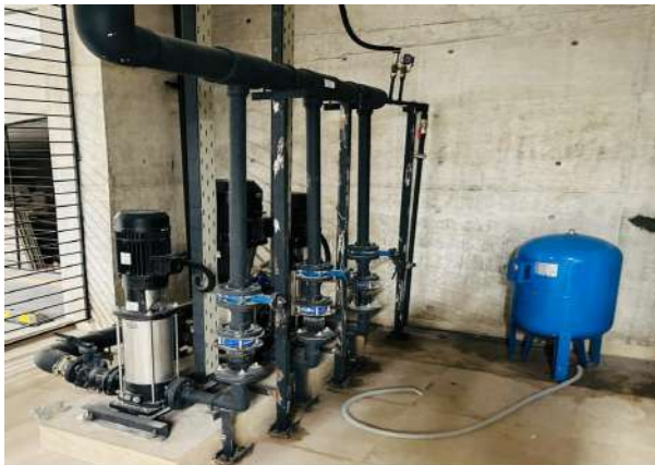
Booster System And WTP
