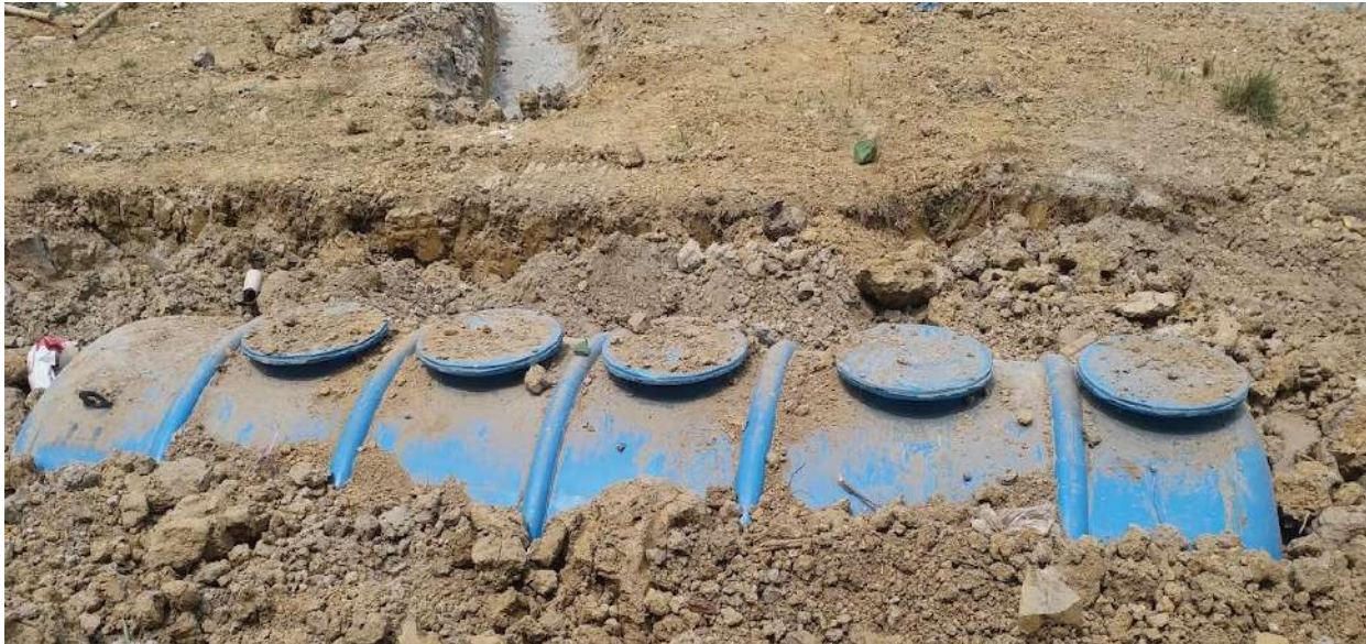
FRP Packed- Sewage Treatment Plant
